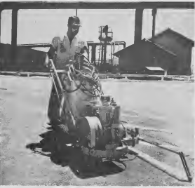
THIS SPECIAL machine is used to paint roadway center lines and can also be used to spray curbing. Tio Giel, tradesman B, is the operator. E MASHIEN uniko aki ta wordé usá pa verf lajuzanan den centro di camina y por wordé usá tambe pa verf acero.
